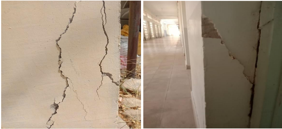
Figure 2: Cracks showing size and orientations in the building.
